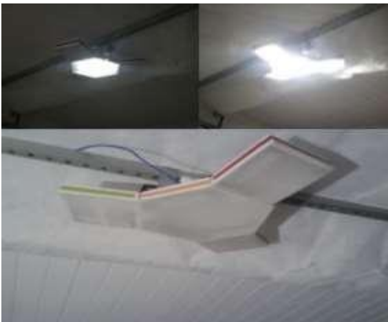
Image 1. LED luminaire installed.
