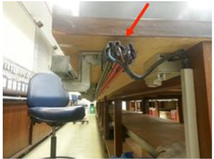
Figure 3: Bottom view of bench and associated electrical bus
